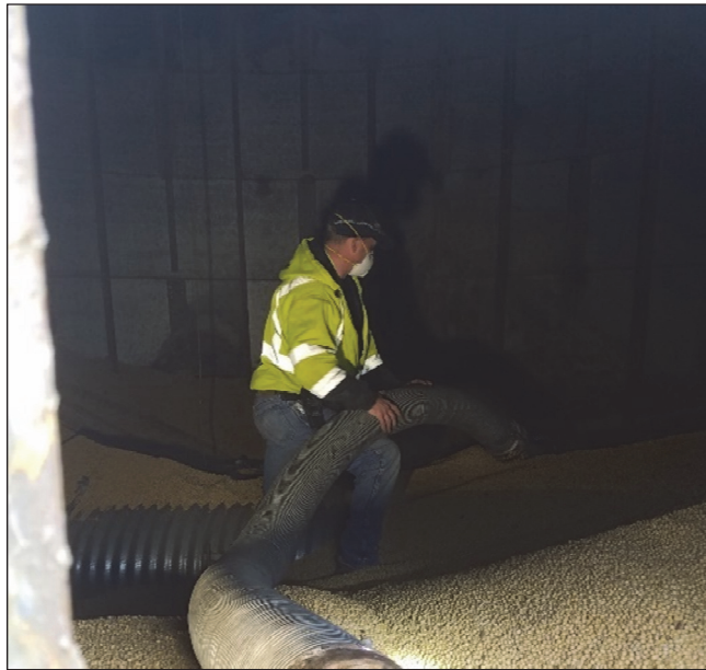
Figure 8. Unsafe example of worker emptying grain bin using grain vacuum while inside bin.
